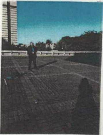
Planning the location and measurements of the concrete base in front of library, S.C.
